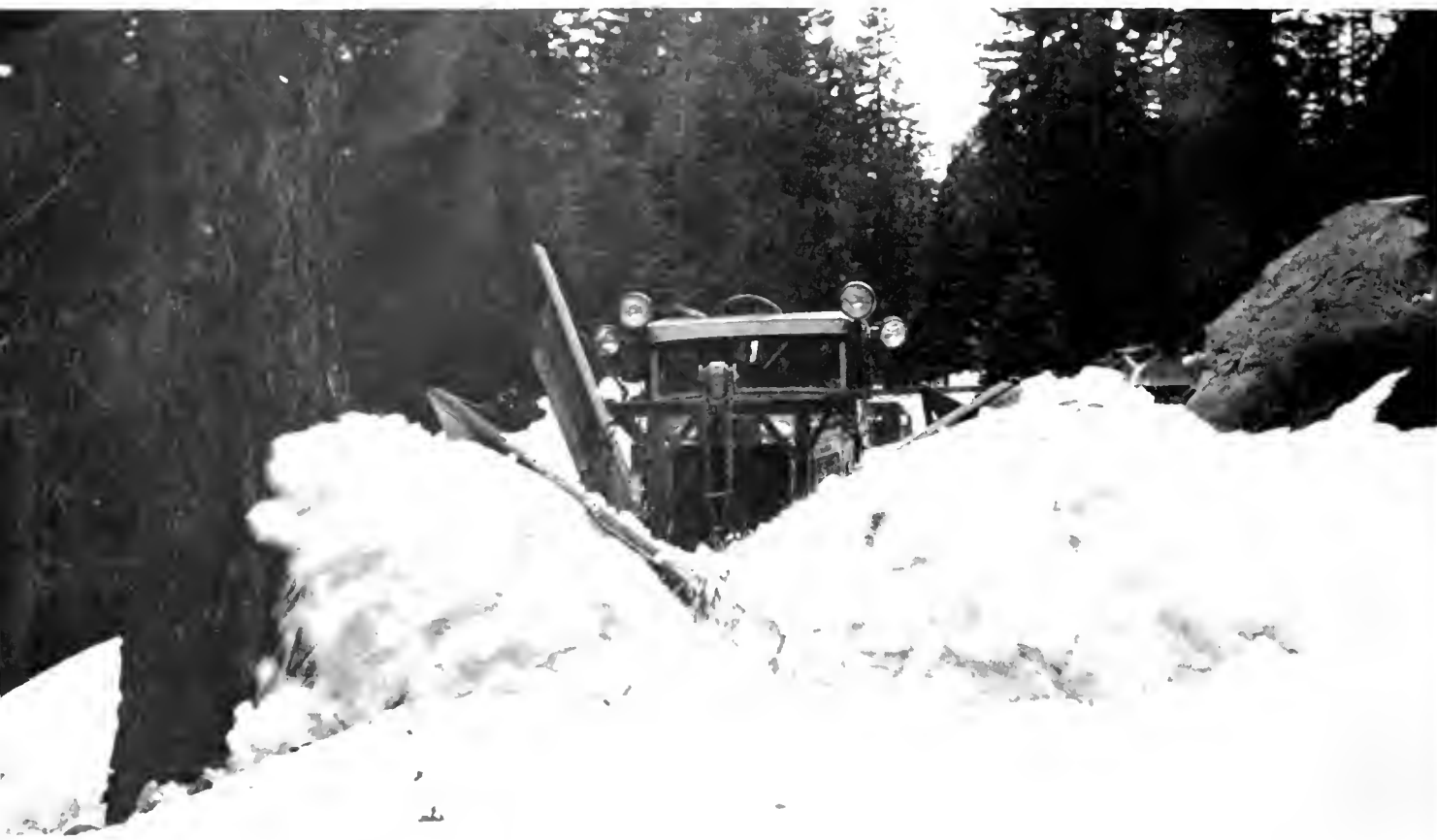
Push plow operating on Meyers grade in March, 1941, in effort to open road for automobile and truck traffic
